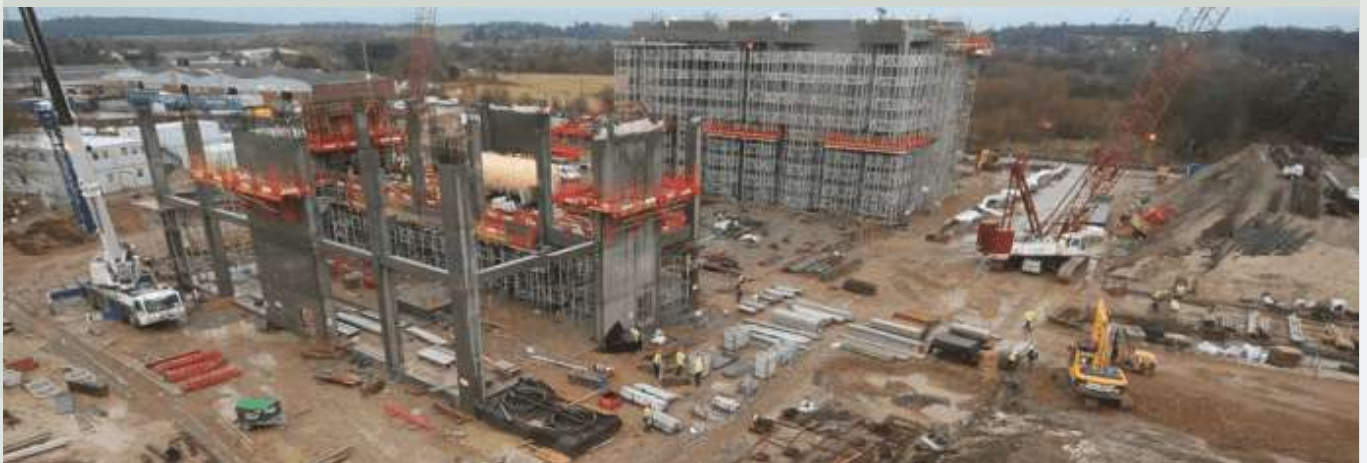
30 LINEAR METRES OF SHUTTABLOC
